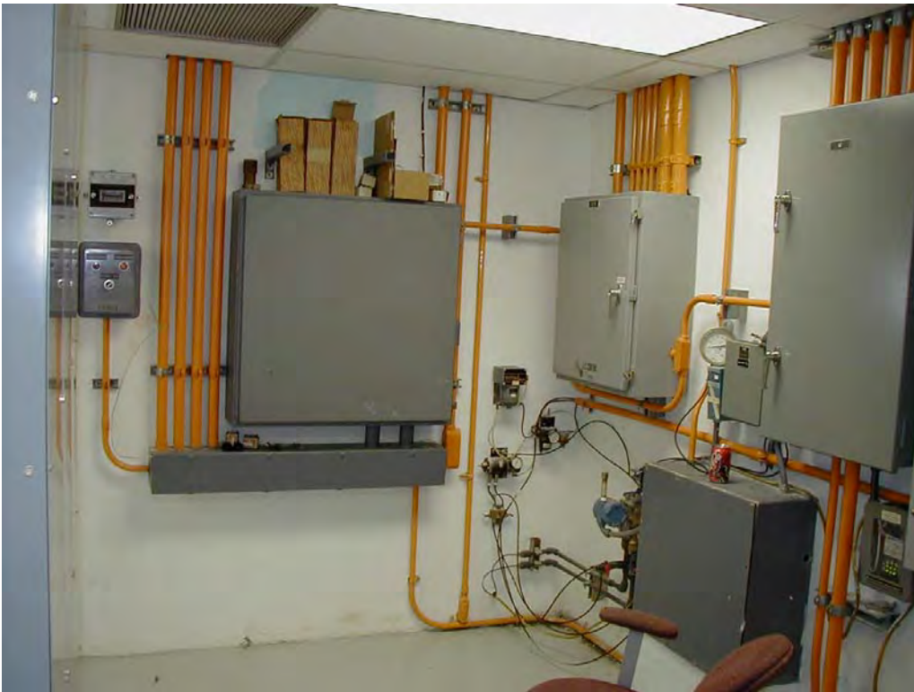
City of Rivera Beach Water Treatment Plant
