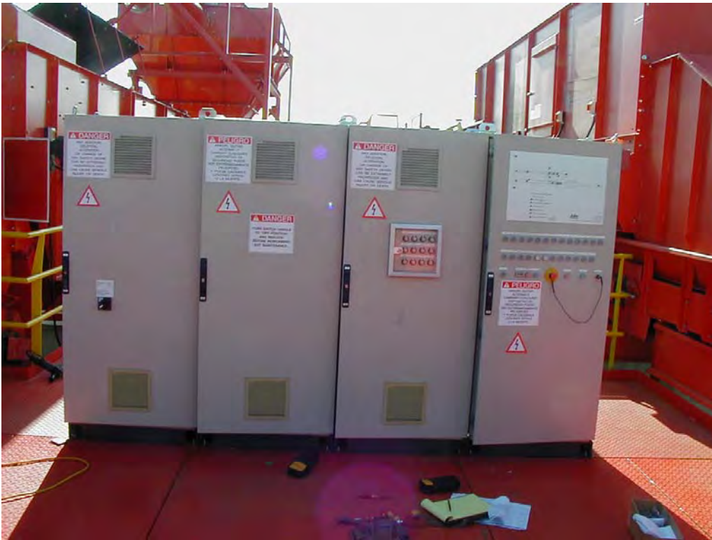
St. Lucie County C & D Facility Switchgear
