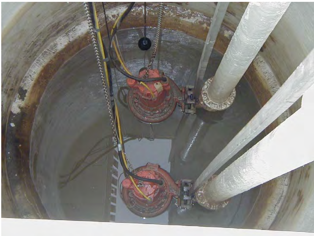
IBIS Lift Station
