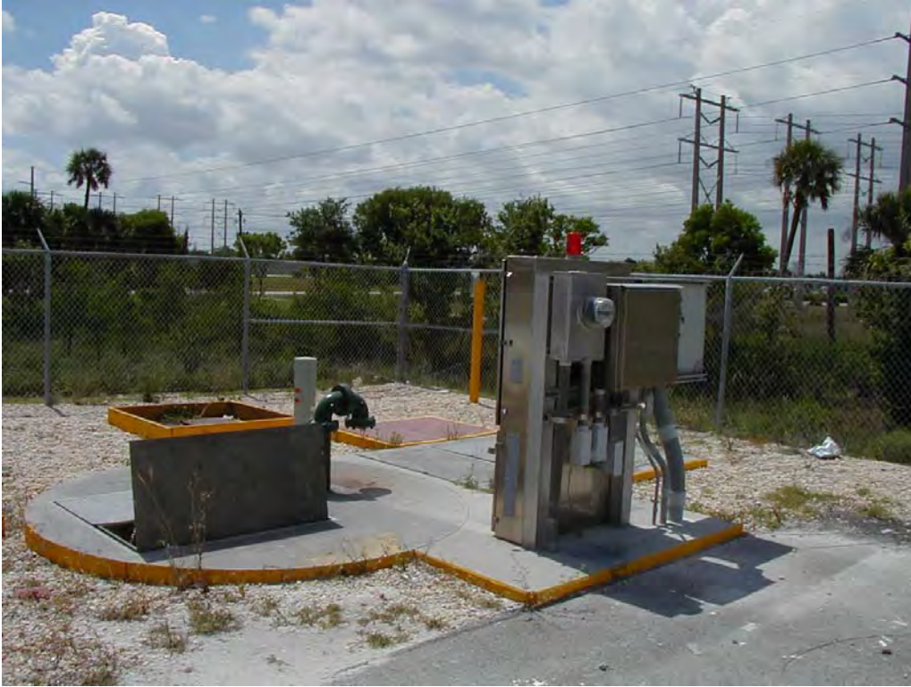
Broward County SWA Leachate Pump Station
