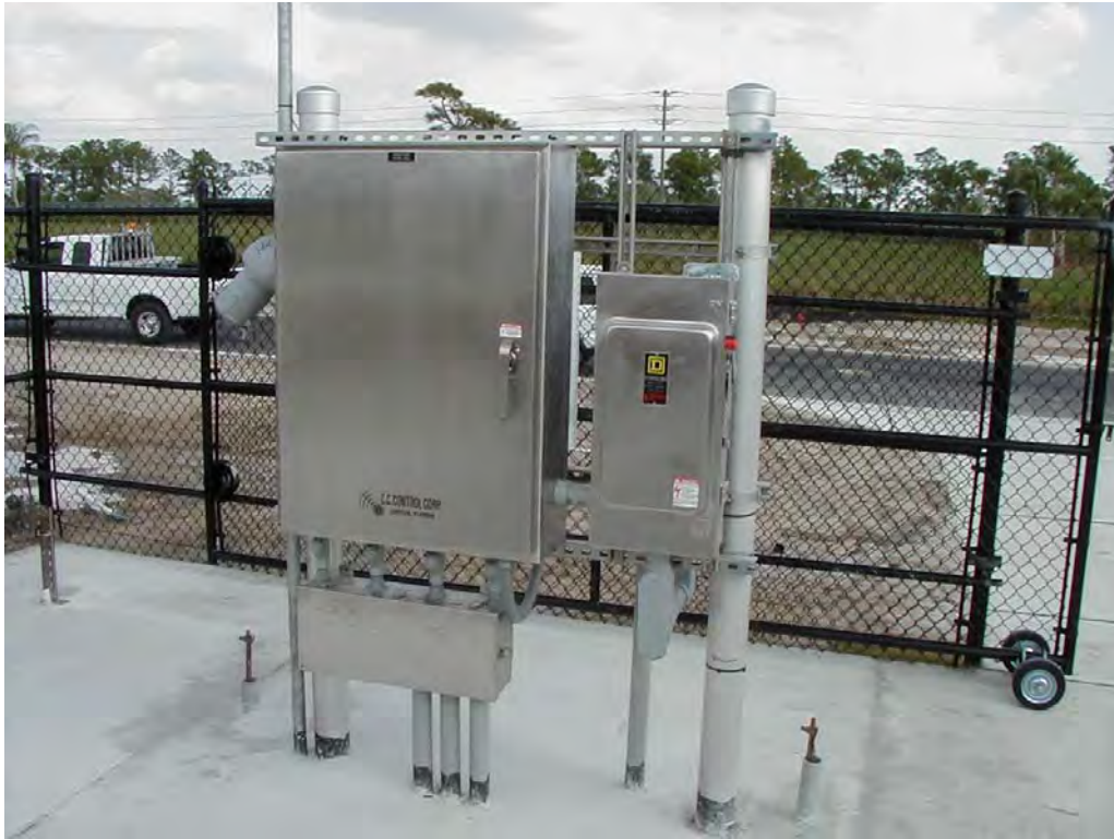
IBIS Lift Station Control Panel
