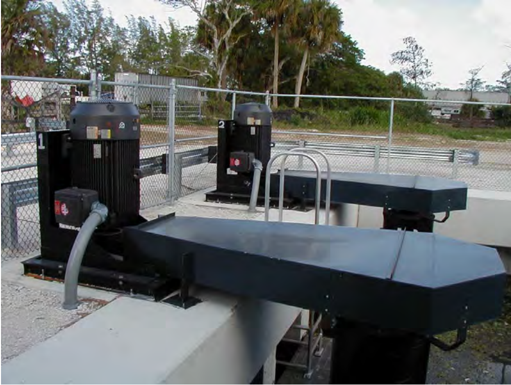
Wellington Pump Station No. 6
