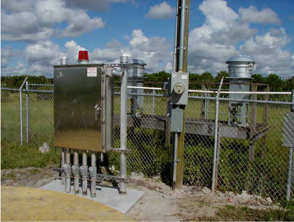
St. Lucie County Landfill Pump Station
