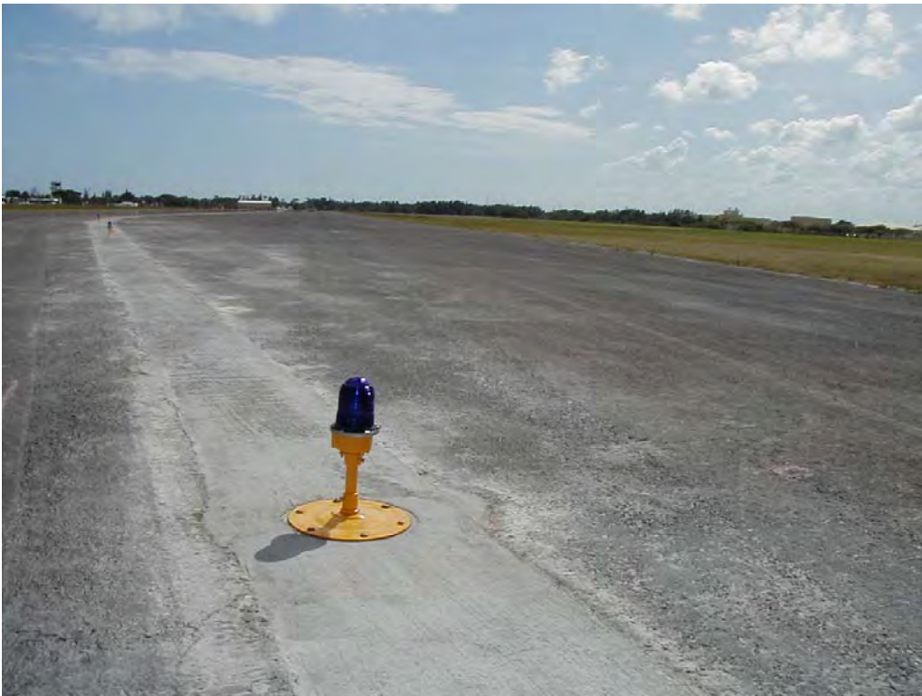
Airport Taxiway Lighting
