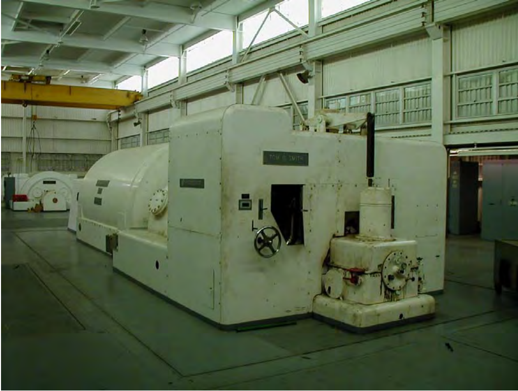
City of Lake Worth Power Plant Generator
