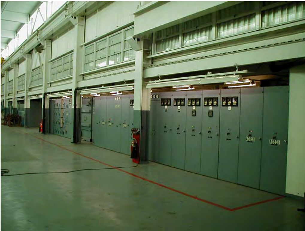
City of Lake Worth Distribution Switchgear
