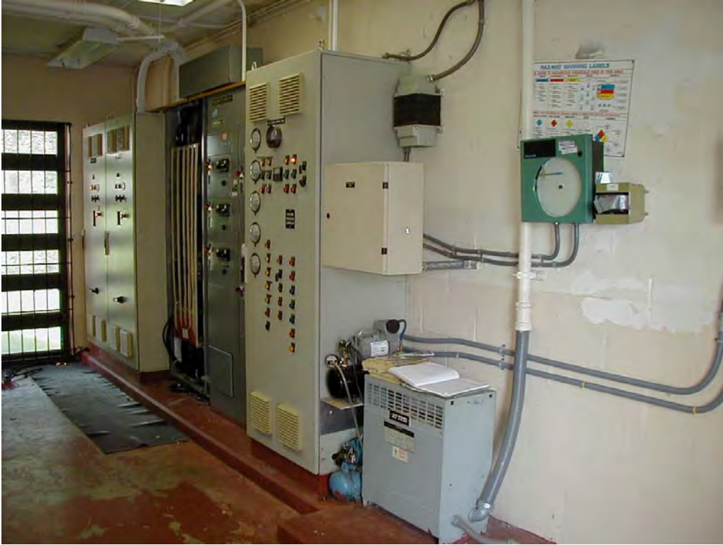
Riviera Beach Master Lift Station
