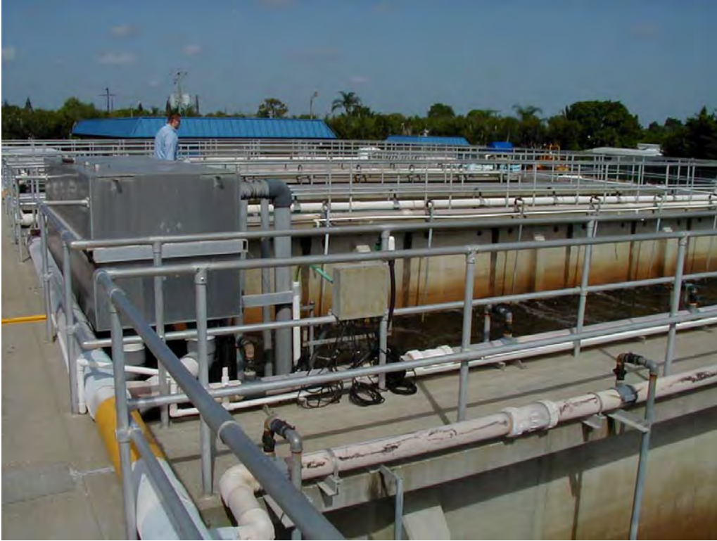
South Martin Regional Utilities WWTP
