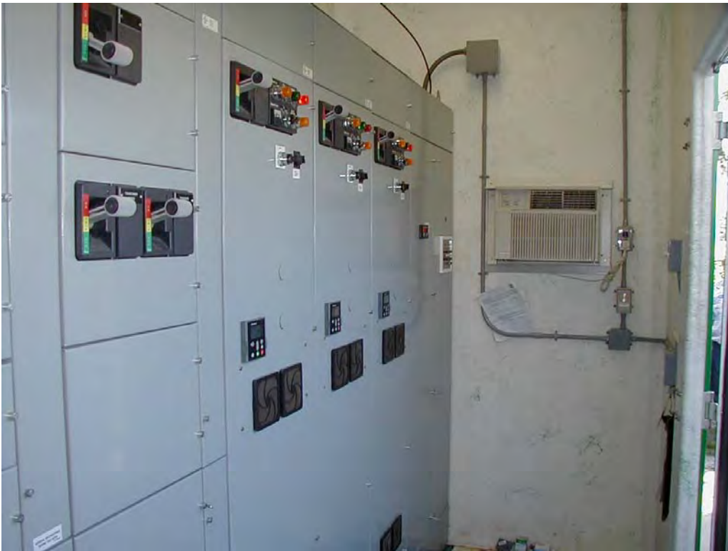
West Palm Beach Master Lift Station
