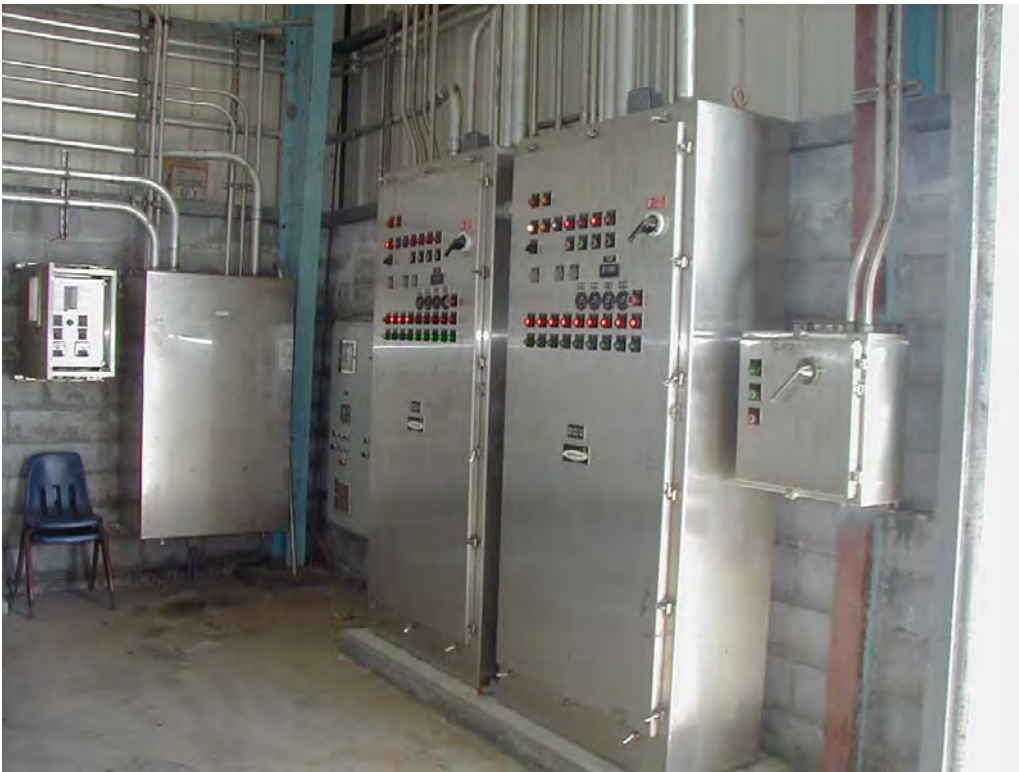
ECRWWTP Truck Loading Control Panels
