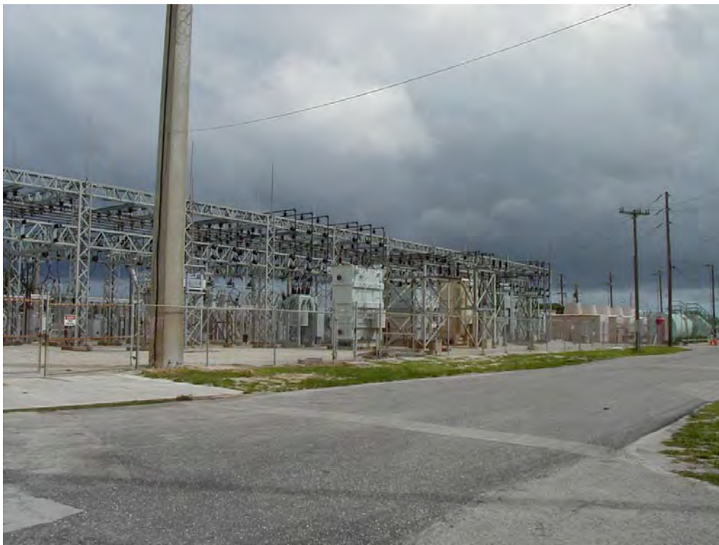
City of Lake Worth Power Substation
