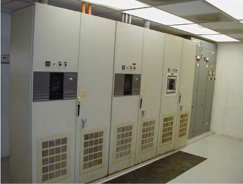
City of Rivera Beach Water Treatment Plant
