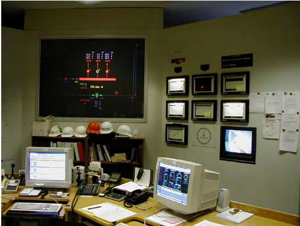
City of Lake Worth Power Generation Control Room
