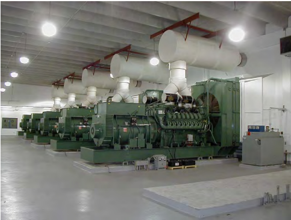
T-Rex Center Power Plant Generators
