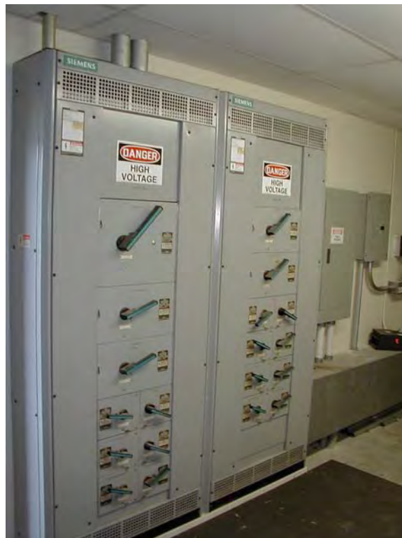
South Martin Regional Utilities WWTP
