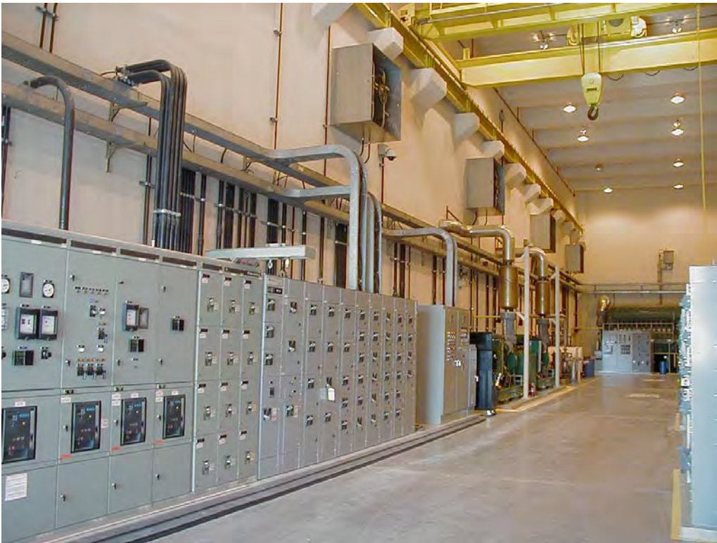
SFWMD Pump Station 319 Switchgear
